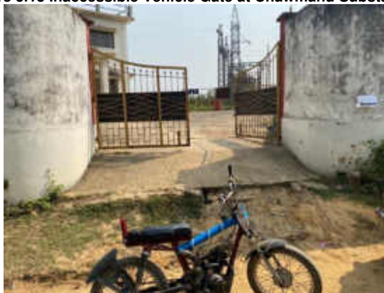
Figure 5.13 Inaccessible Vehicle Gate at Chawmanu Substation
