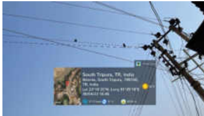
Figure 3.9 Photograph of Existing Covered Conductors in Tripura
