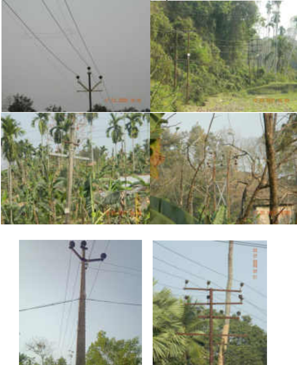
Figure 3.8 Existing Overhead Lines in Tripura with Uncovered Conductors
