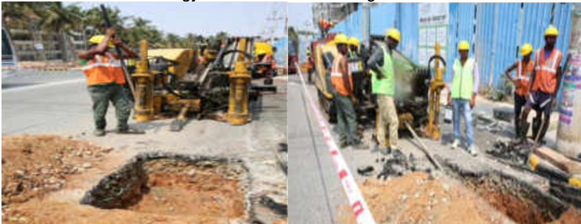
Figure 3.21 Representative Photographs of Drill Rig and Entry Pit in Trenchless Technology for Installation of Underground Cables
