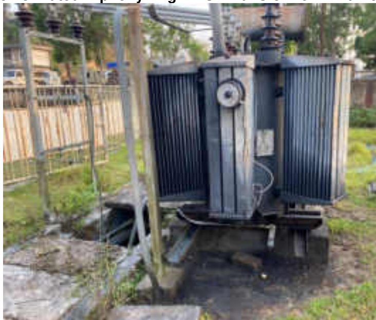
Figure 5.8 Polychlorinated Biphenyl High Risk Transformer in Damchara Substation
