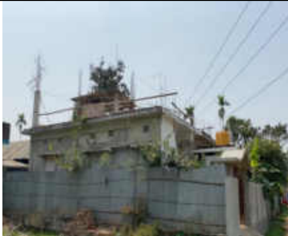
8. 33 kV UG from Grid Sub Station to College Tilla Substation showing electrocution risk for people on rooftop. This line to be moved to UG
