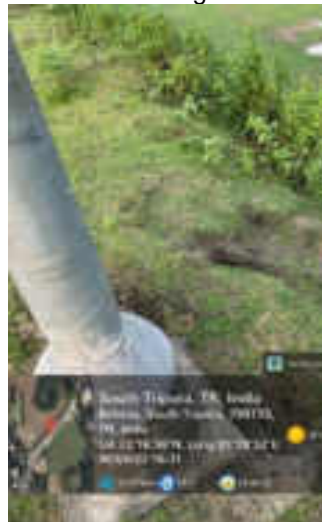
Unstable pole on eroded roadside along Chittamura Feeder line, South Tripura Source: ADB TA Consultant
