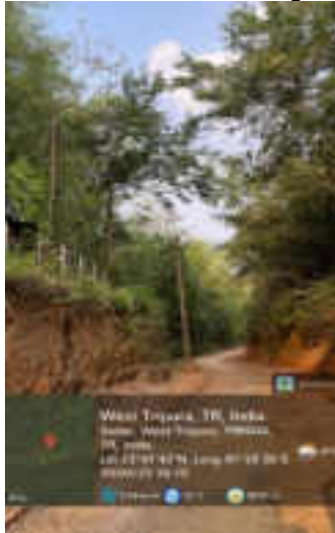
Washed away pole foundation due to road cutting in Ananda Nagar feeder line, West Tripura
