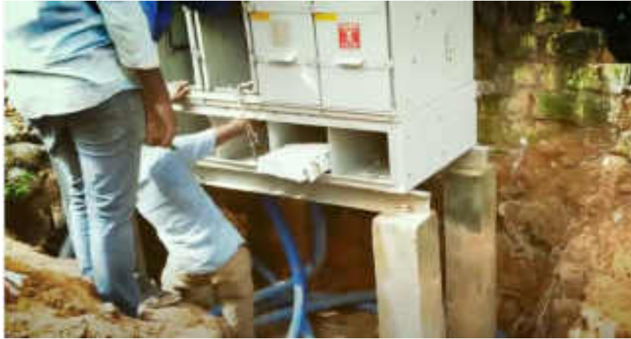
Figure 3.22 Representative Photograph of Ring Main Unit Installation
