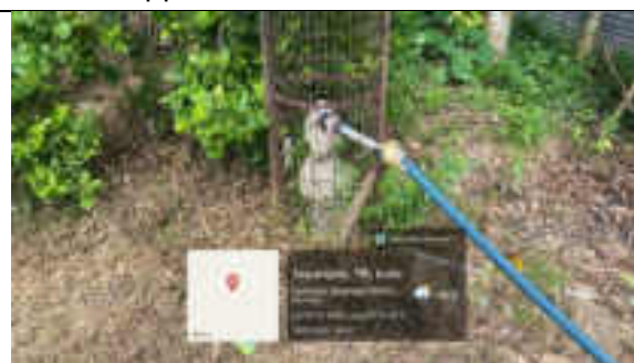
Bore well with pump in Manikyanagar village, ESD Boxarnagar
