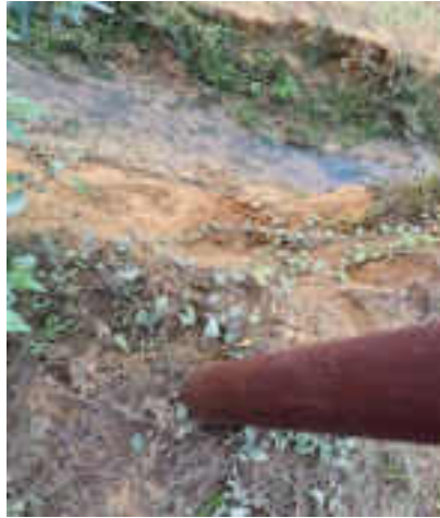
Washed Away Foundation of Distribution Line Pole During Monsoon Season in Gomati District
