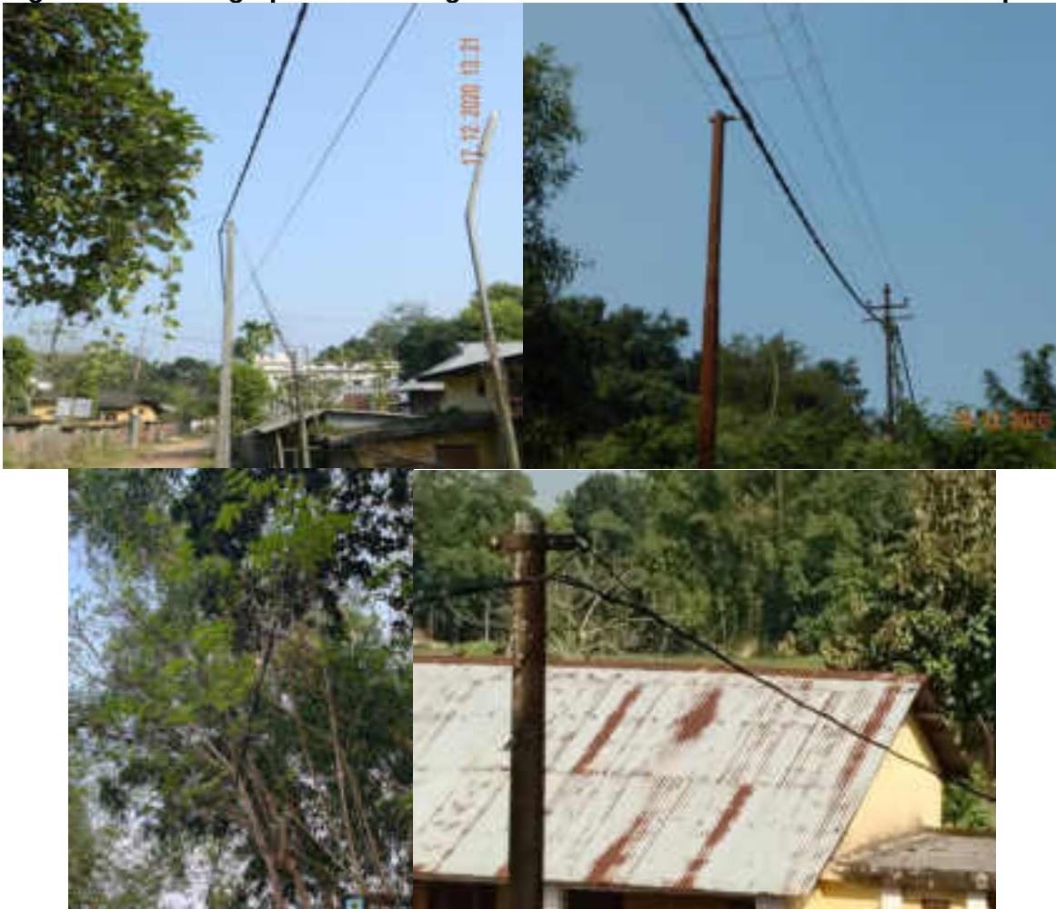
Figure 3.10 Photographs of Existing Low Tension Aerial Bunched Cables in Tripura
