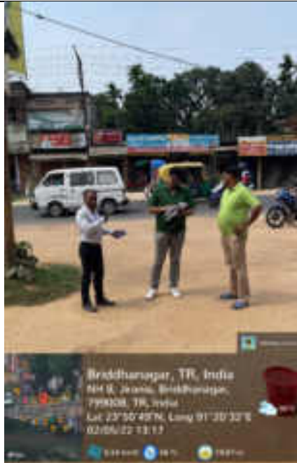
Consultations in the Bodhgangnagar to Adarsha Colony Substation New 33kV Underground line
