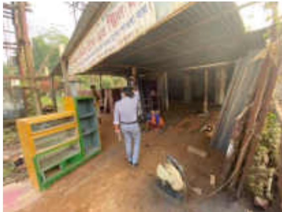
3. Shops adjacent distribution transformer and within ROW (66KV Gokulnagar Substation to 33kV Madhupur Substation) - potential risk from cable fault, transformer burst, fire etc.
