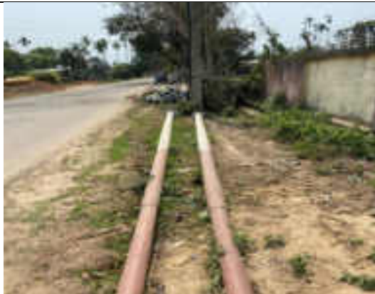
1. 11 kV Degalbagh Feeder to bifurcate existing Raghna Feeder route with poles stored along road – potential for vehicle/pedestrian accident
