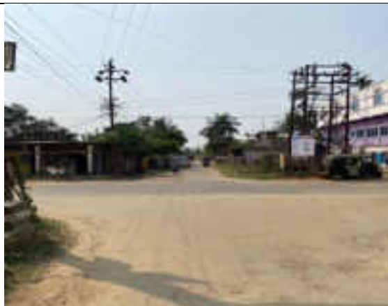
5. 11 kV Degalbagh Feeder to bifurcate existing Raghna Feeder route showing crossing with a hospital (white building) - during construction congestion, storage of material and pole dismantle/new may cause H&S risk to locals
