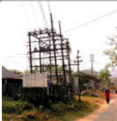
Ground mounted transformer without fence on main road with shops adjacent near Gokulnagar Madhupur distribution line route, Sipahijila District
